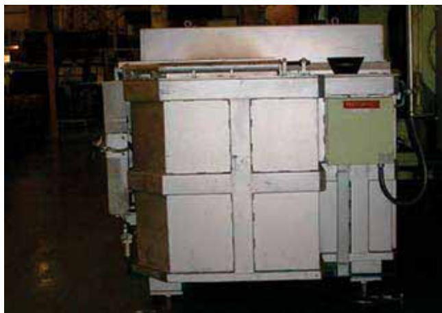
Figure 2 — Electric immersion holding furnace.
