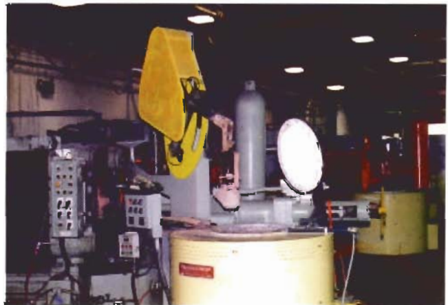
Figure 1: Energy efficient solid state electric resistance furnaces in a die casting facility with robotic pouring.
